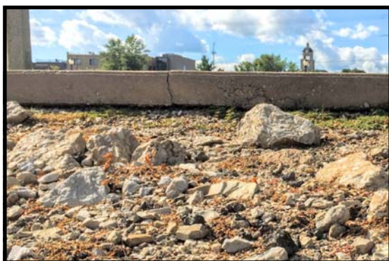
Erosion Beginning to Undermine Harbor Sidewalk
