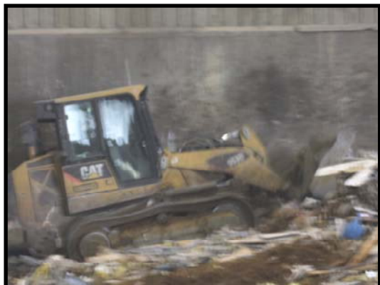
Track Loader that is to be replaced
