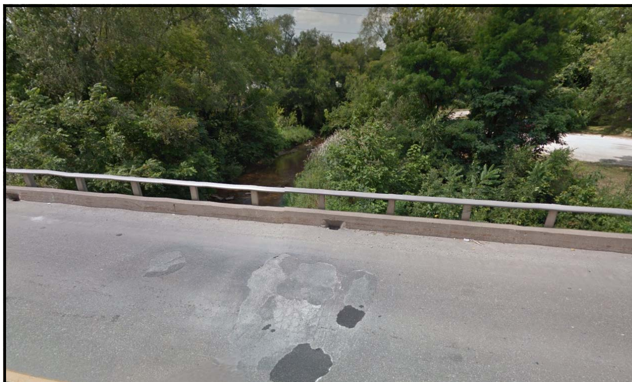
Scoring at the 2nd Street Bridge
