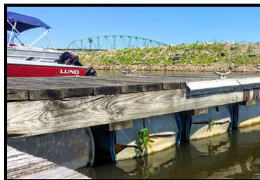
:Floats Deterioration at the Long Dock
