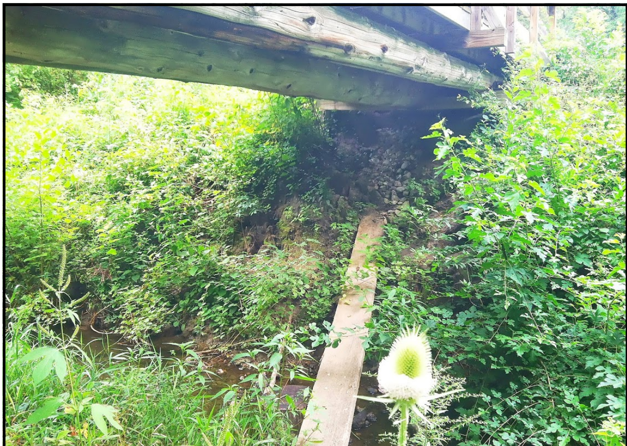
Erosion at Fuller Park
