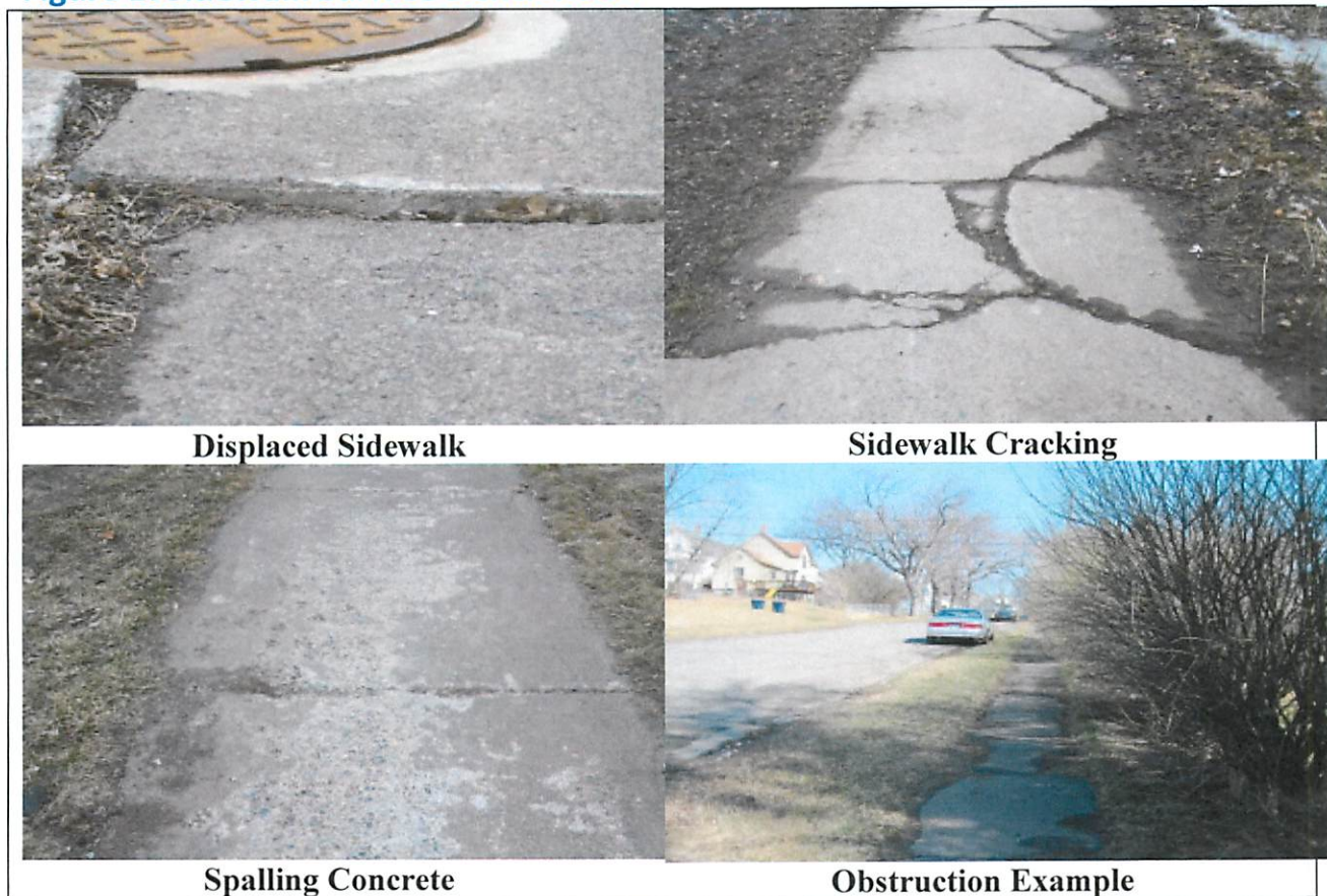
Figure 1: Sidewalk Surface Deficiencies 5
